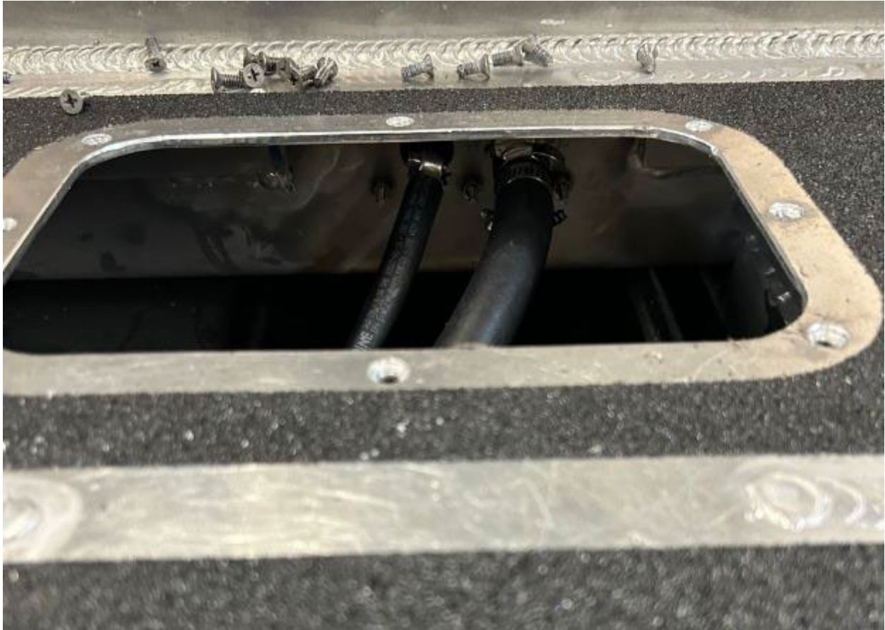
Figure 8: With the hatch ring removed the vent hose connections are accessible for inspection.
